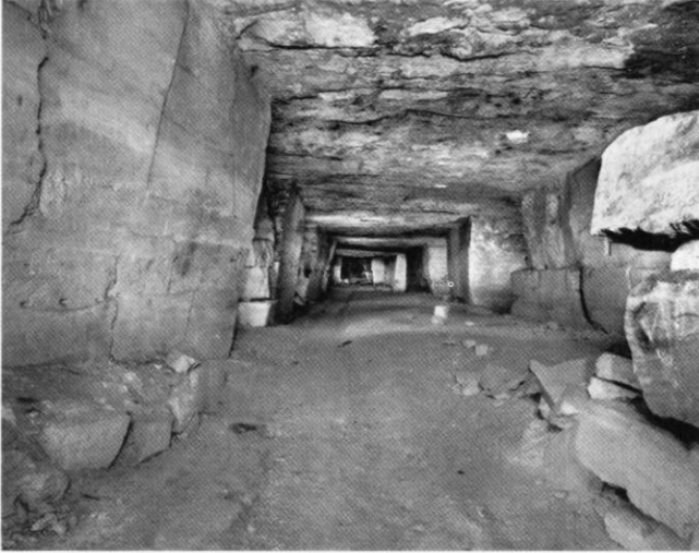
The wide span of unsupported roof found in much of the quarry indicates that large blocks of good quality stone have been removed. Photo Nick Catford
